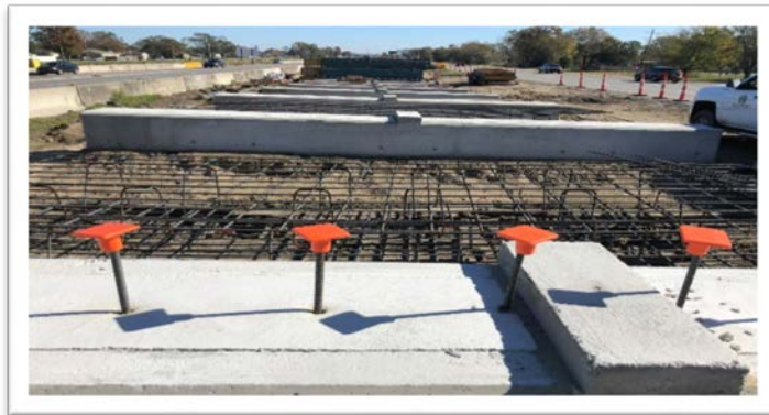
Ramp G Caps
